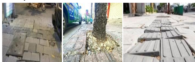
Figure 3. Sidewalk paved with interlocking tiles showing unevenness and displacement (Source: Author)
