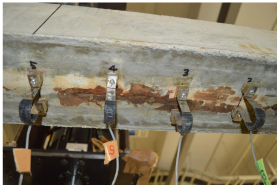
Figure 10. Crack gauges at the middle of the beam
